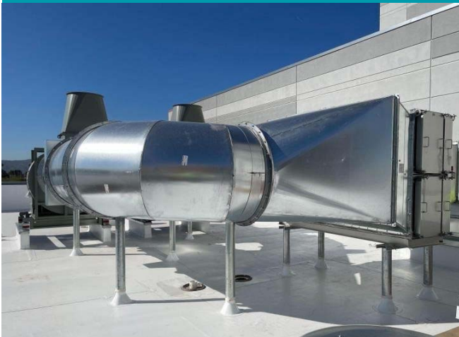
Level 2 Roof Sally Port Exhaust Duct
