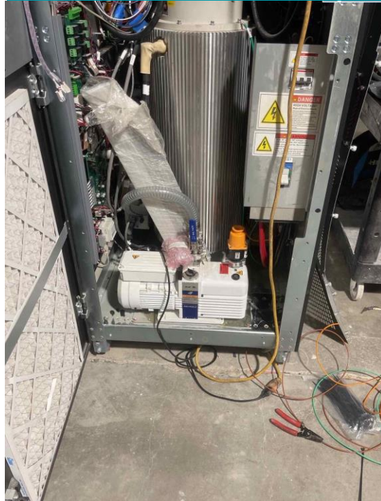
Basement Essential Elec. Room
